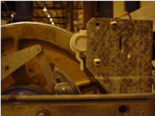
OS in the Tripped Position
